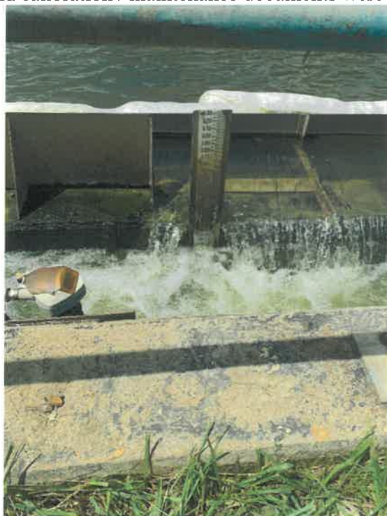
Staff gauge at Outlet 001 to verify ultrasonic flow meter.
